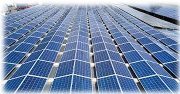
Distributed / Centralized PV Power Stations
