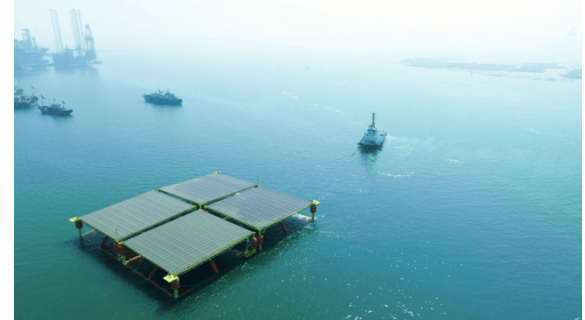
China, 400 kWp Souce: CIMC Raffles
