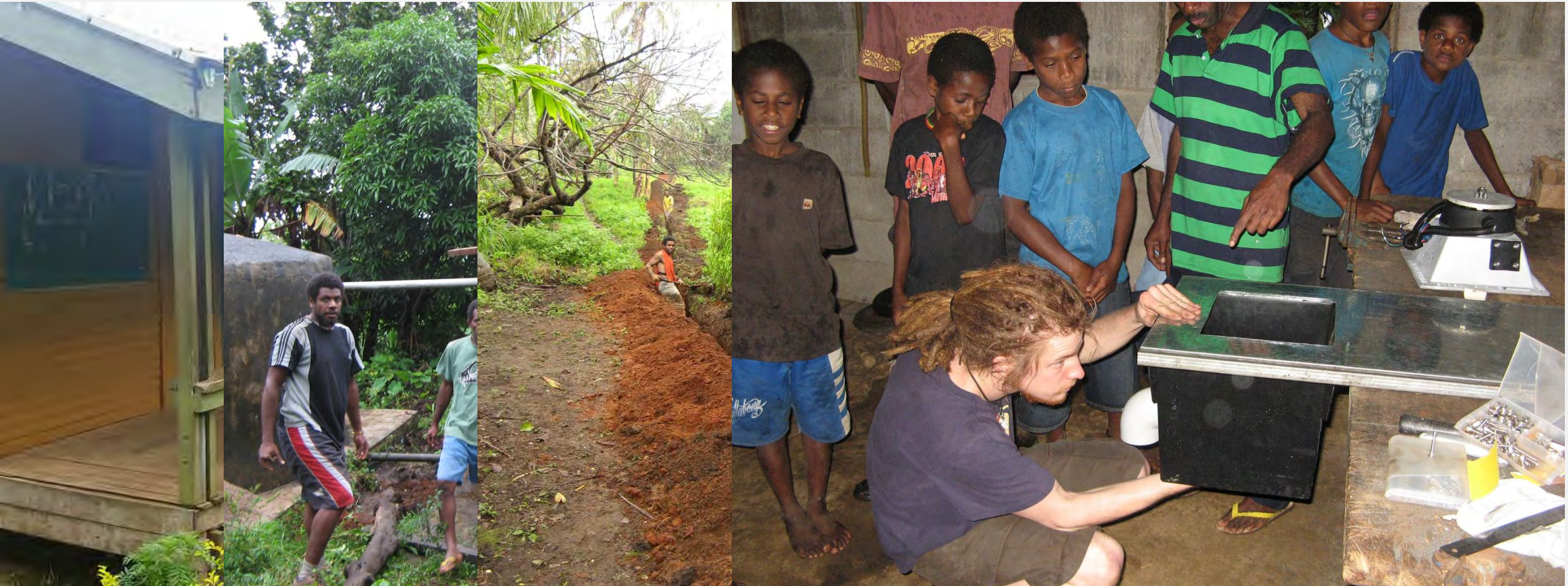
Hydro power from existing water supply line
