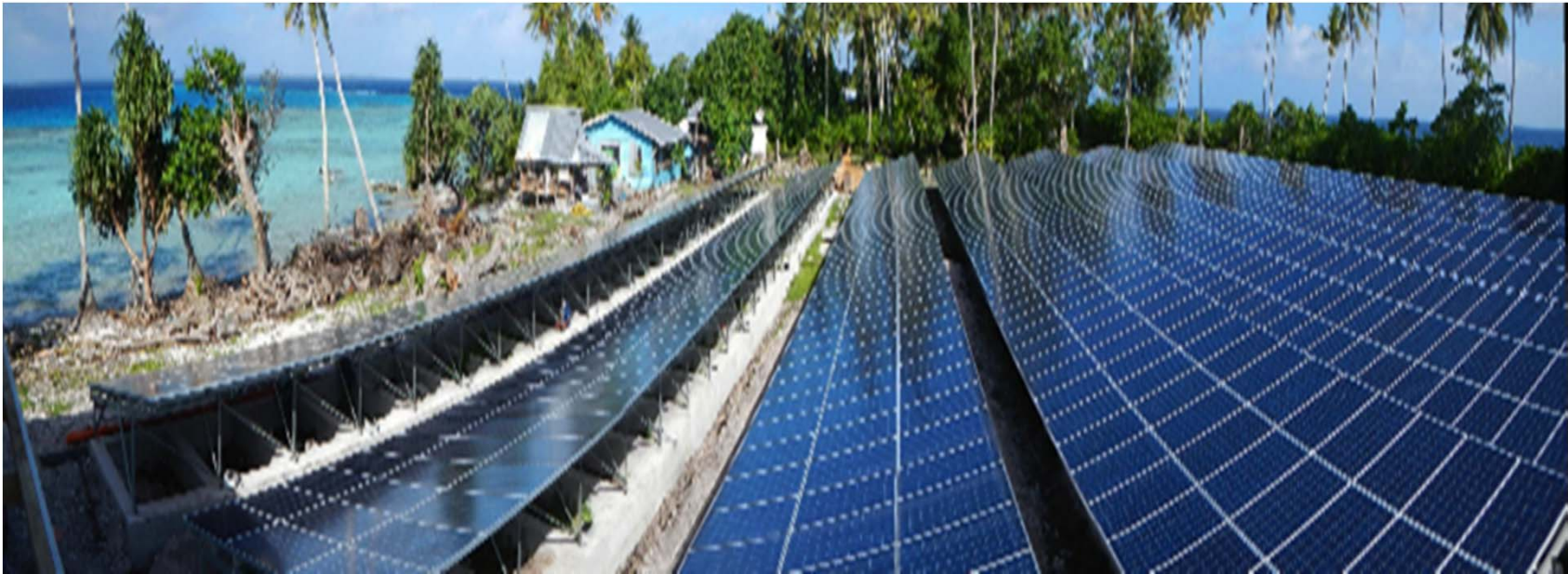
Tokelau PV system. Photo: IT Power
