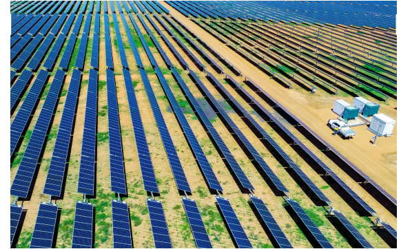
Nevertire Solar Farm (132MWDC)
