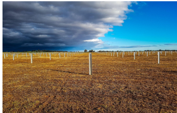
Parkes Solar Farm (66MWDC)
