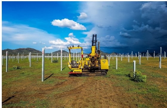
Hamilton Solar Farm (138MWDC)
