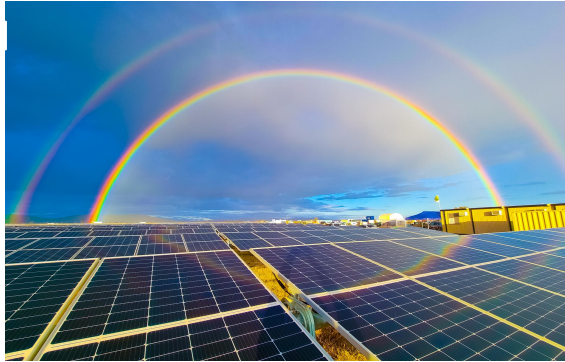
Gunnedah Solar Farm (146MWDC)
