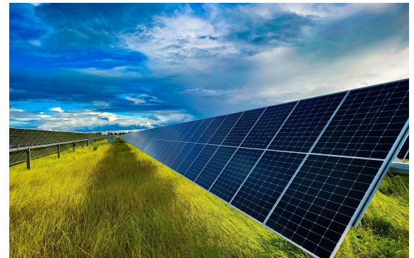
West Wyalong Solar Farm (107MWDC)
